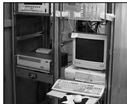
Monitoring systems in trailer in Vermont.
